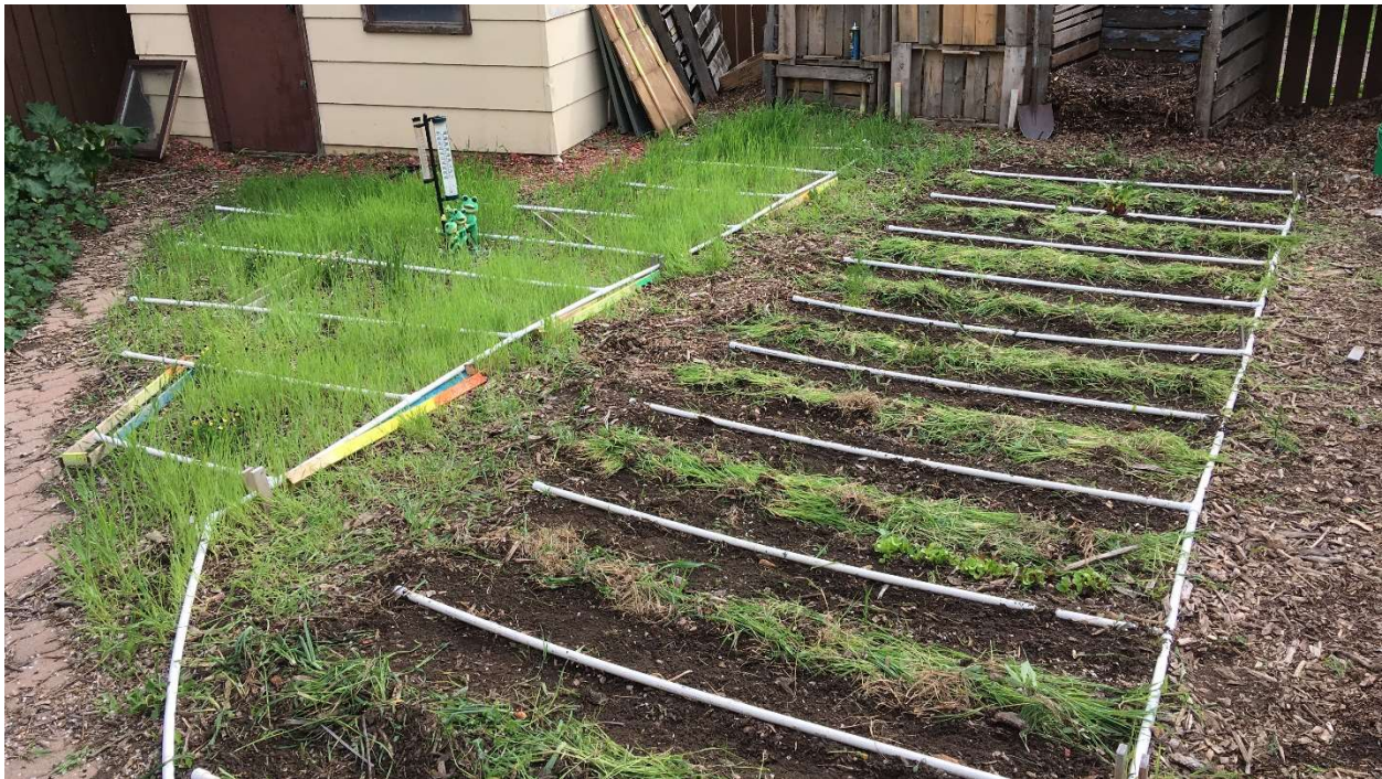
PVC drip irrigation system
